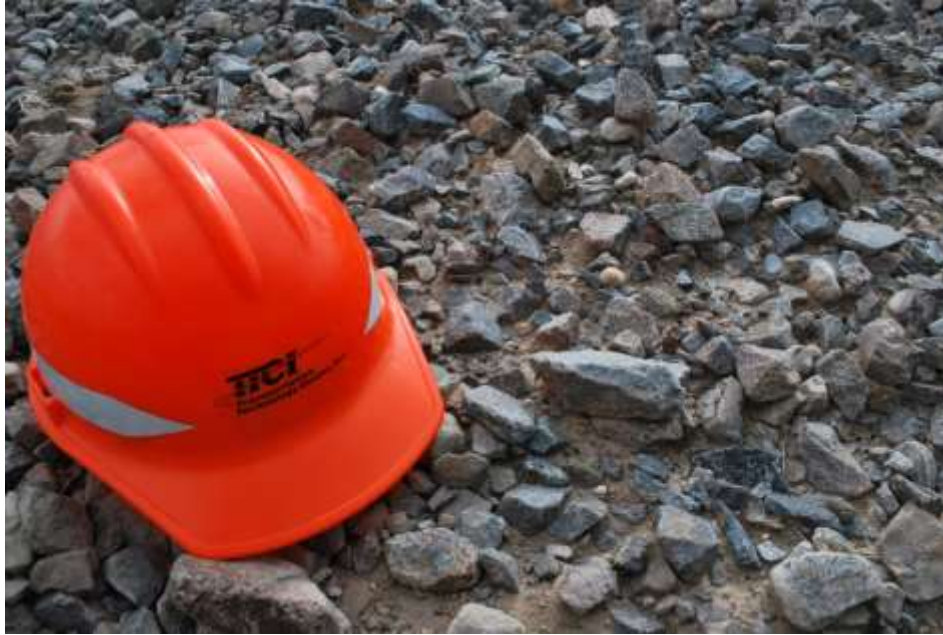
Figure 1.3 An example of fouled ballast
